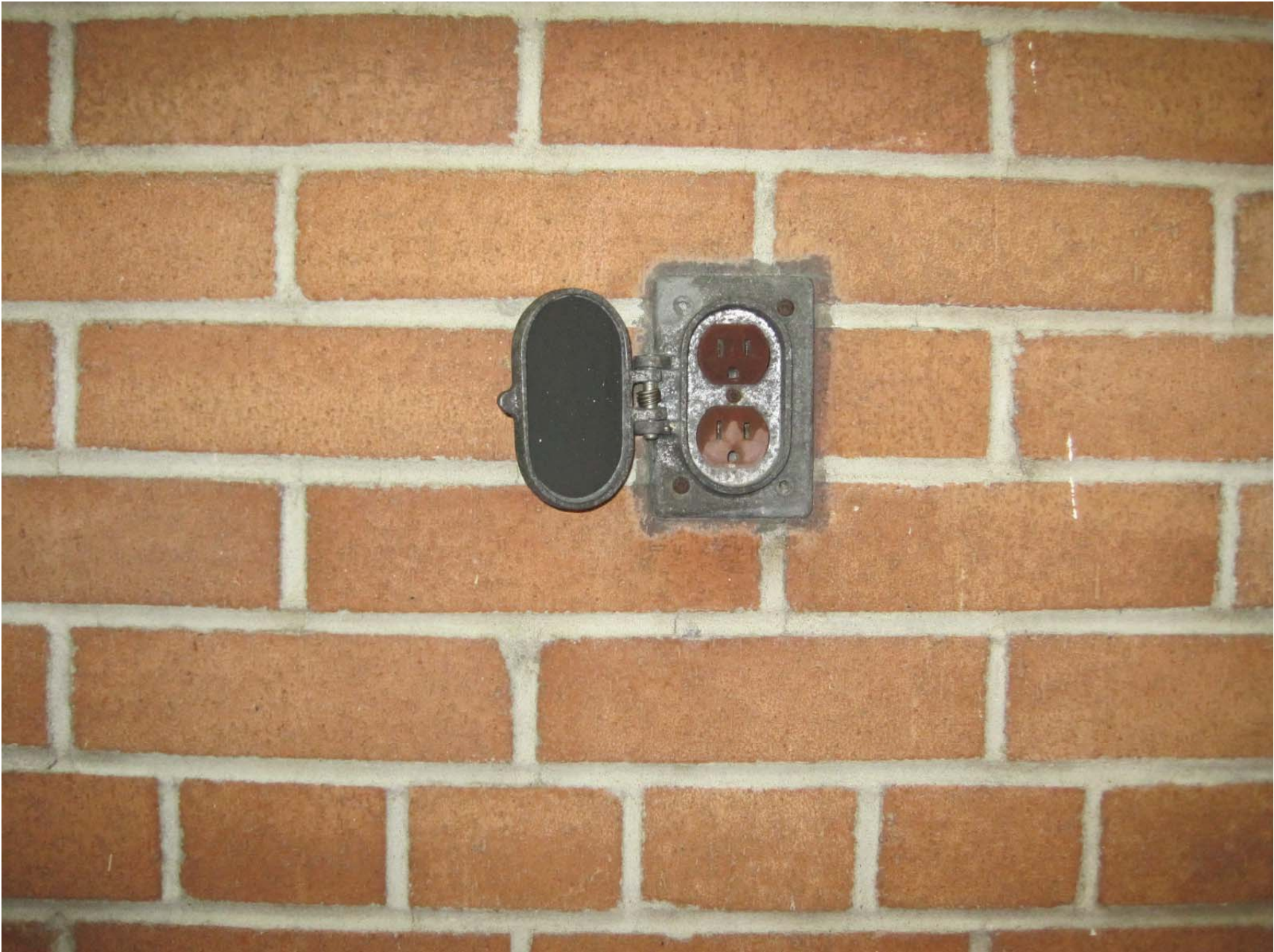
CLOSE UP SHOT OF ELECTRICAL OUTLET
