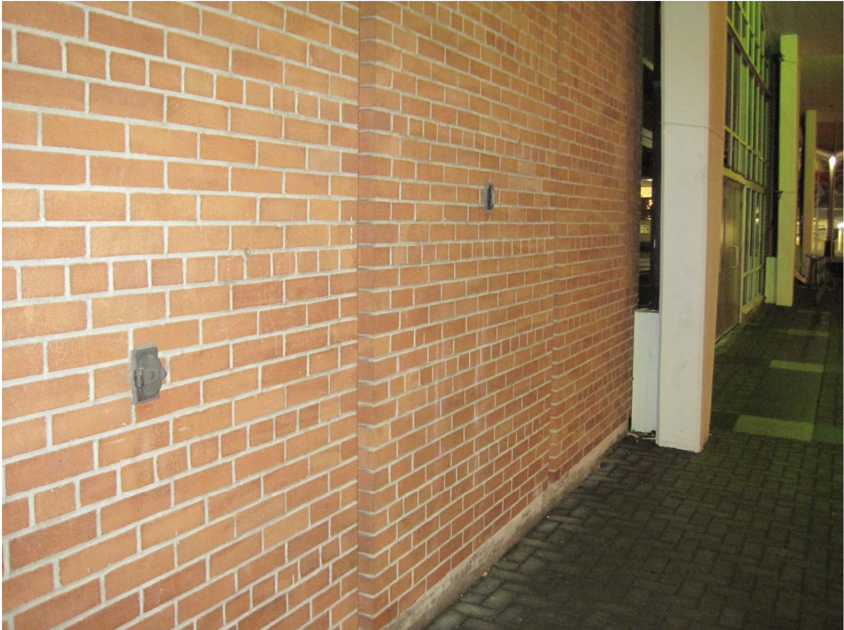
ELECTRICAL OUTLETS TO THE WEST OF THE MAIN ENTRANCE
